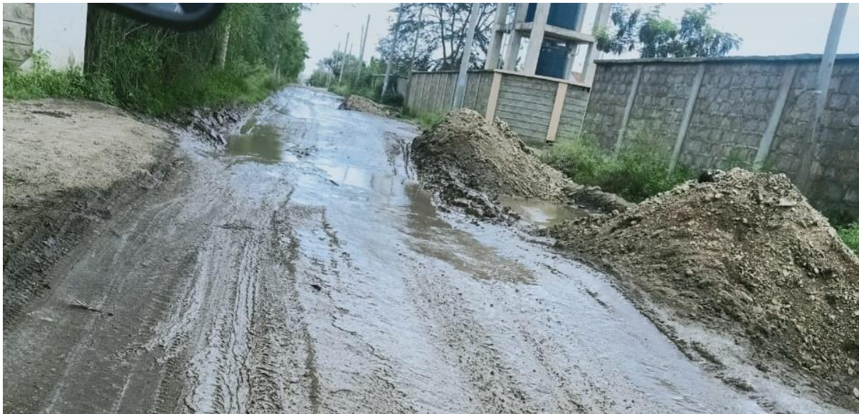
Figure 3-44: Poor roads in Milimani
