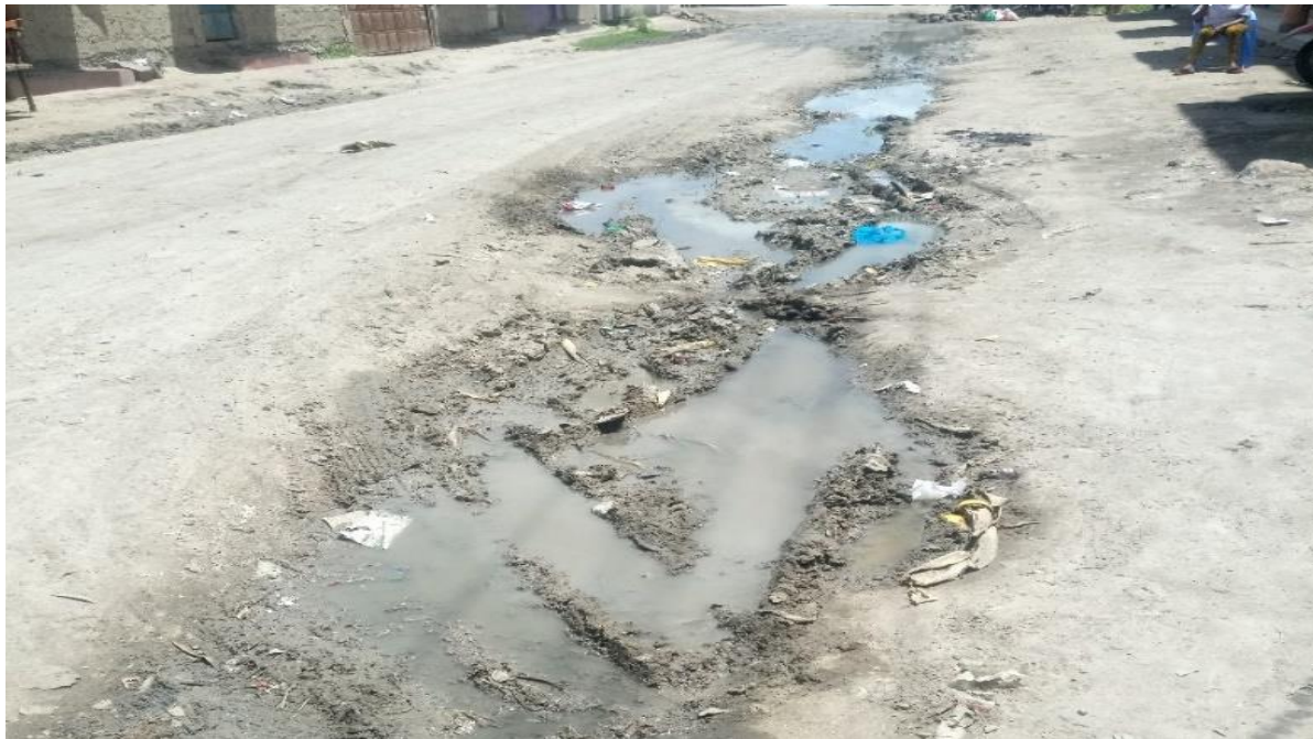
Figure 3-82: Example of a poor storm water drainage
