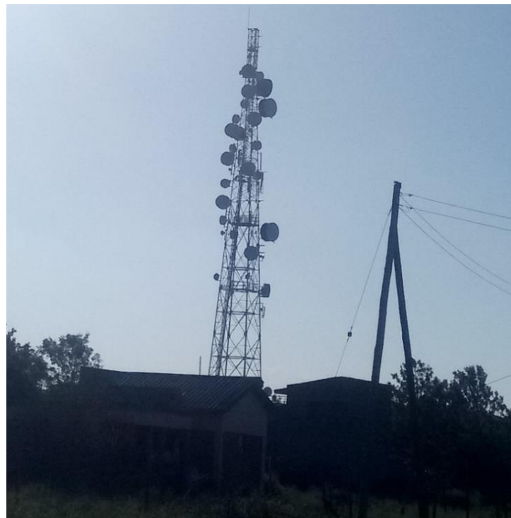
Figure 3-74: Safaricom communication mast at Safaricom
